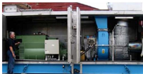
Fig. 4.5. Gas turbine generator set Dresser-Rand of the power of 1.5÷2 MW in ISO container body ( www.powercity.ru )
